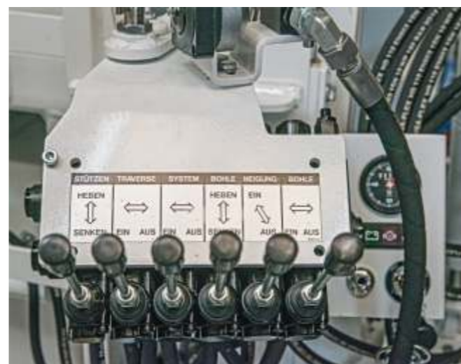
additional control element to regulate the height for connection with trucks.
